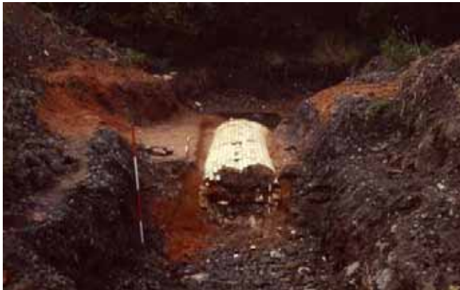
GIW Tr4 Machine dug trench (TR4) revealing large white brick air intake approximately 1 m in diameter.
