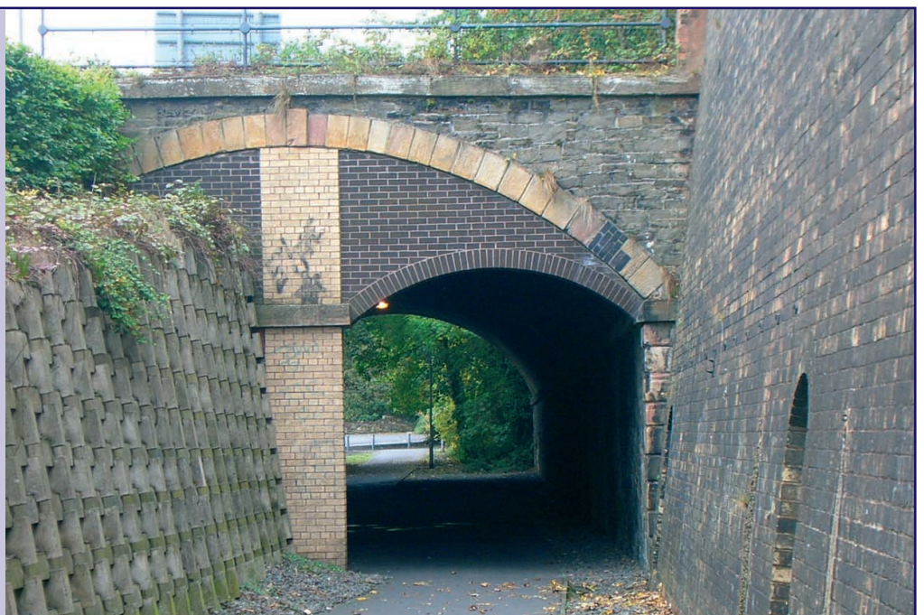
Ladhopevale, Galashiels, looking north: The new line will run along the existing footpath.
